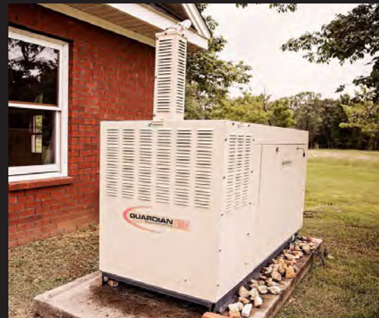
Whole House Generator
